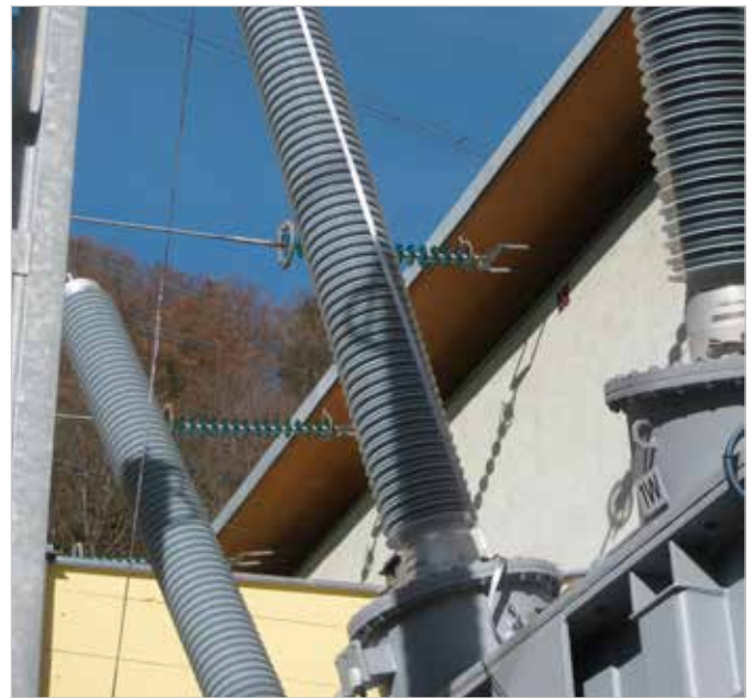
Figure 6. Example of shortest-braid connection concept: measurement cables (black) are connected to the bushing terminal and the grounding braid to the terminal and bushing flange
