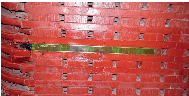
Figure 2. Measuring coil in PCB technique installed on the stator tooth
