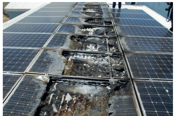
Figure 13. The consequence of fire on photovoltaic system, example [9]
