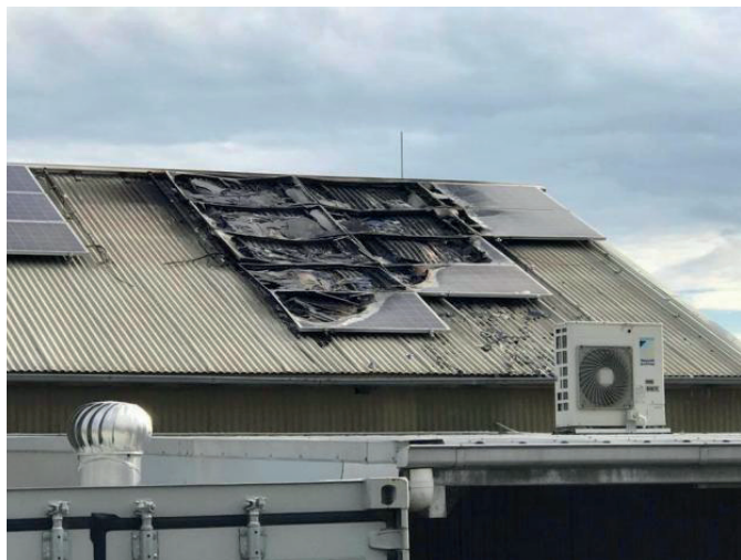
Figure 14. The consequence of fire on photovoltaic system, example, [10]
