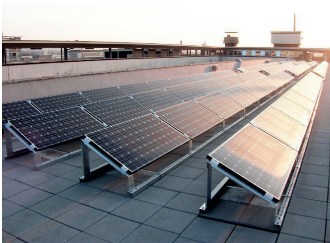
Figure 1. PV panels on the flat roof, picture source Končar d.d.
