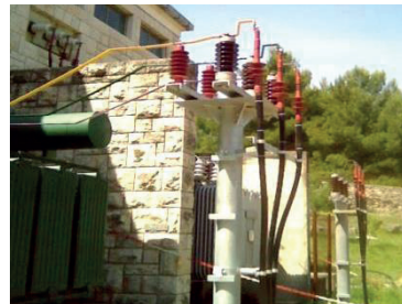
Image 8 Bracket of support insulators, surge arresters and cable terminals on a 35 kV side of the power transformer
