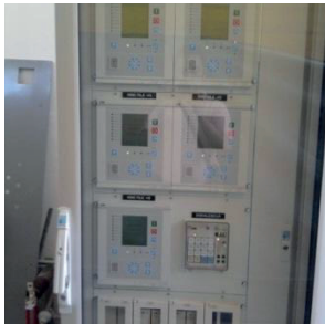
Image 10 Protection cabinet of the 35 kV plant
