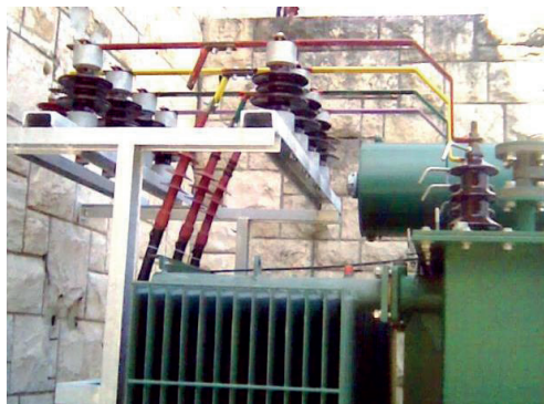
Image 9 Bracket of support insulators, surge arresters and cable terminals on a 10 (20) kV side of the power transformer
