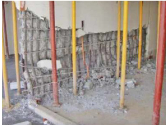
Figure 1. Wall damage - earthquake in Chile
