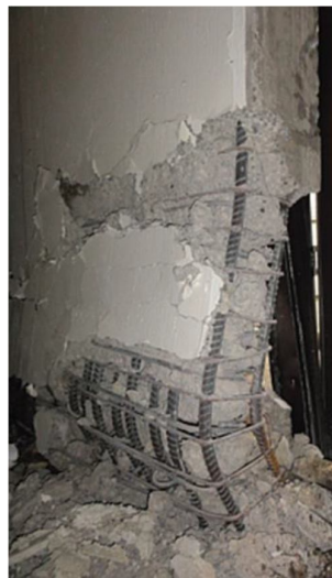
Figure 2. Wall damage - earthquake in New Zealand
