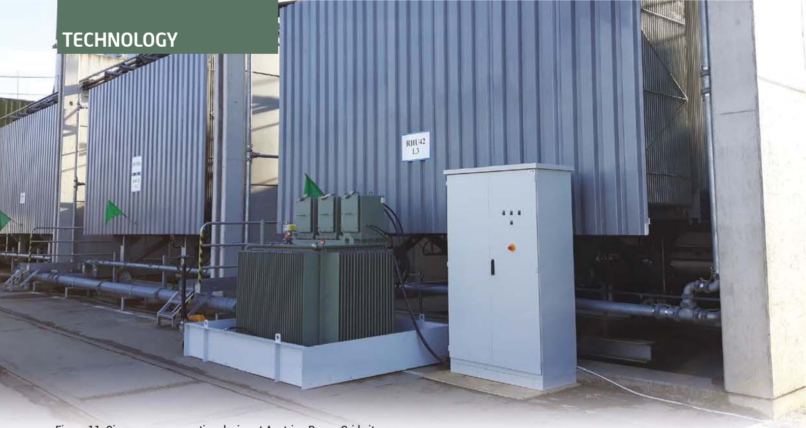
Figure 11. Siemens compensation device at Austrian Power Grid site
