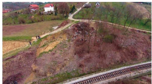
Fig. 16. Picture of landslide taken from UAS
