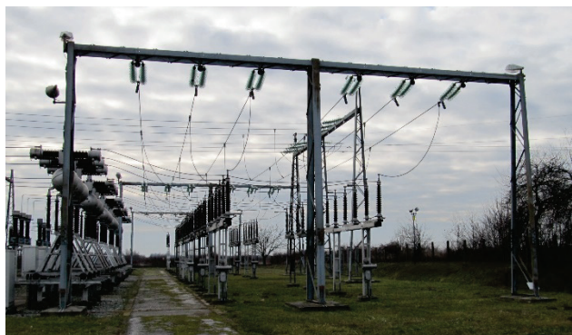
Figure 1 Wire busbars in S/S 110/35 kV Valpovo 2
