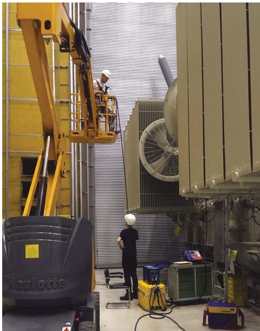
Figure 4. One-time connection of the three-phase transformer test system to perform all electrical tests according to Table 1
