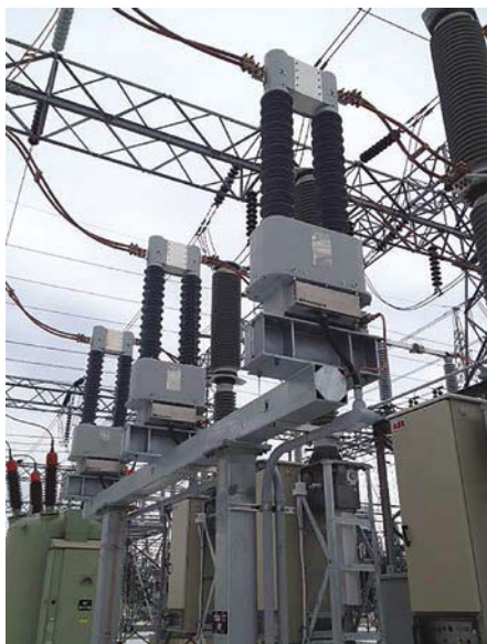
Figure 4 – 115 kV dry type current transformer installation in Western Canada
