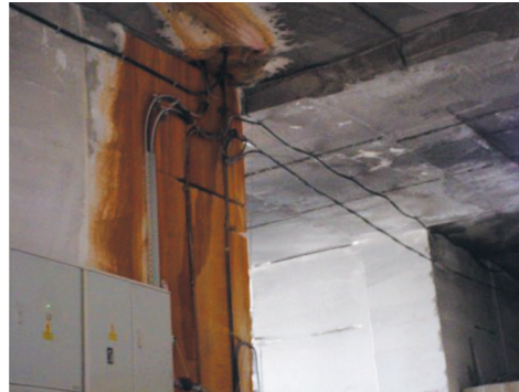
d) energetska stanica
