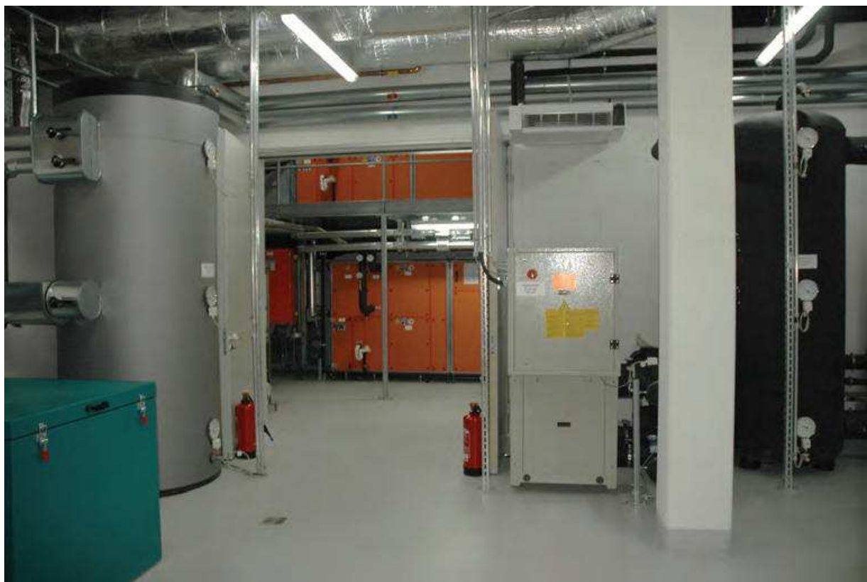
Figure 3. Technique room of the Central Art Depot
