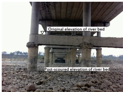
Figure 2 The vertical and horizontal pile foundation scour photo of Minjiang River Bridge No. 3
