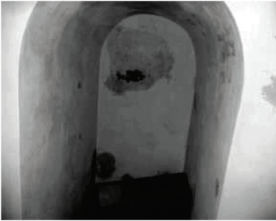
Figure 2 Accumulation of moisture in the external wall of the temple building during the annual operating cycle.
