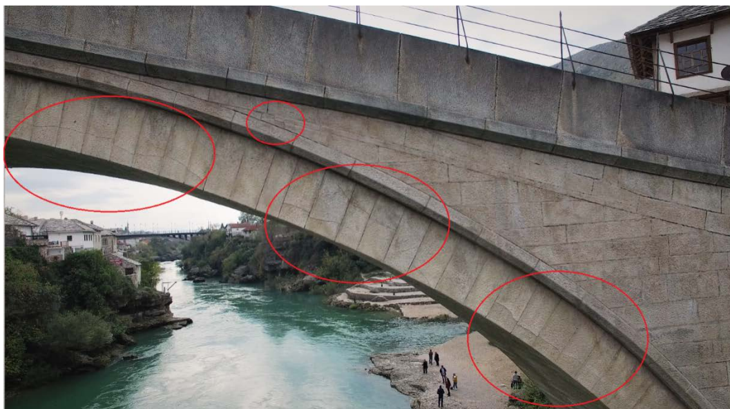
Figure 10. Cracks on the upstream side of the arch in 2018
