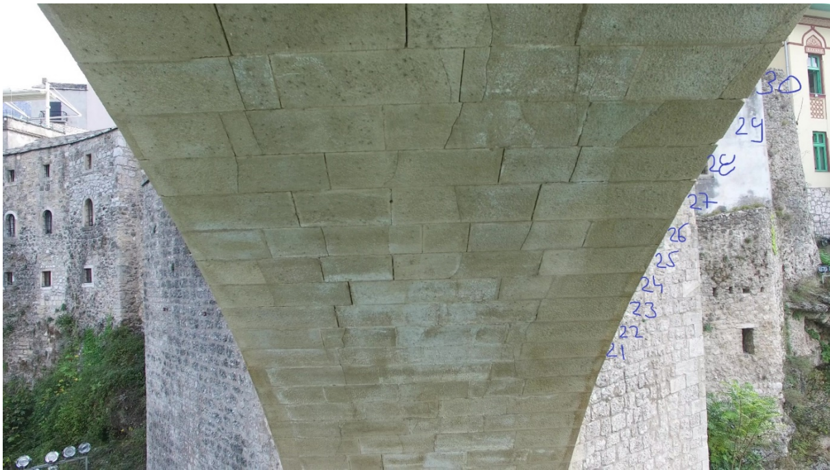
Figure 13. Cracks on the bridge intrados east side, 2018
