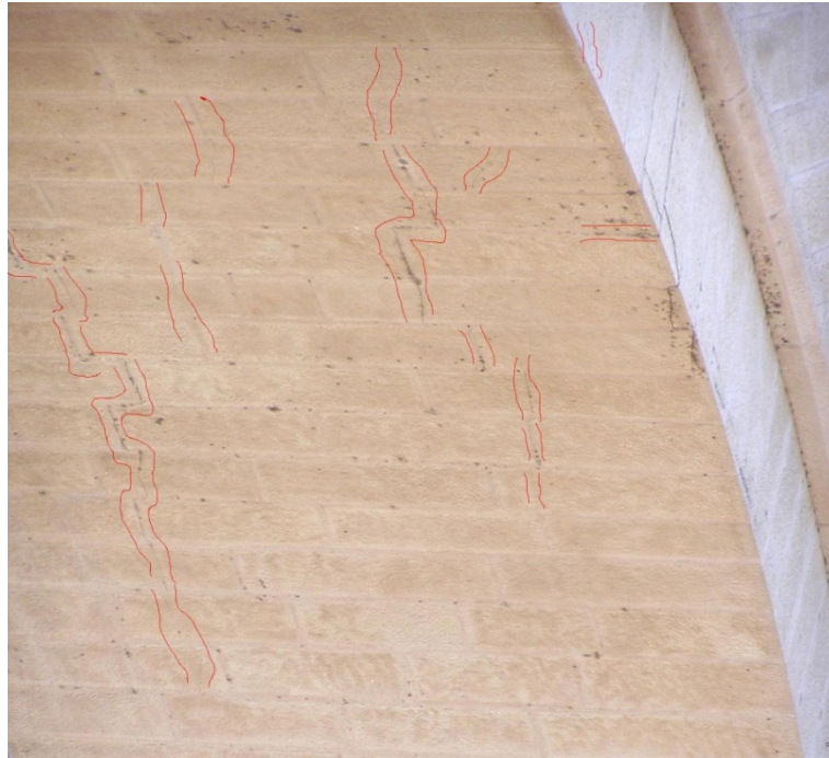
Figure 2. Cracks on the bridge intrados on 9 November 2008.
