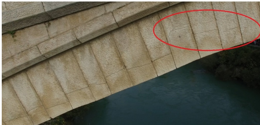
Figure 9. Cracks on the downstream side of the arch from 2013 and 2018. Visible new cracks to the right of the benchmark
