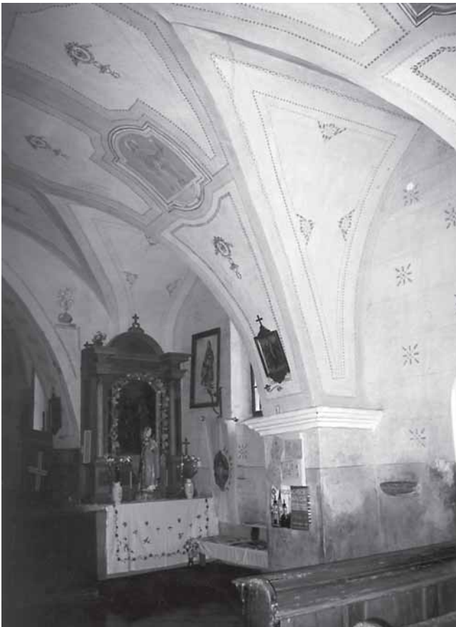
6. Velika Erpenja, susvodnica u svodu broda (foto: D. Botica) 6. Velika Erpenja, ribs in the ceiling of the nave
