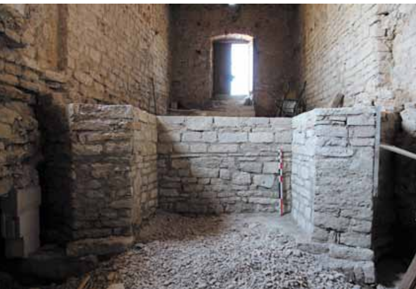
sl. 37. Djelomično rekonstruirani zidovi W 25, W 44, W 45 i W 65 tijekom restauracije (A. Milošević). Fig. 37 Reconstruction of walls W25, W44, W45 and partly W65 during the restoration campaign (A. Milošević).
