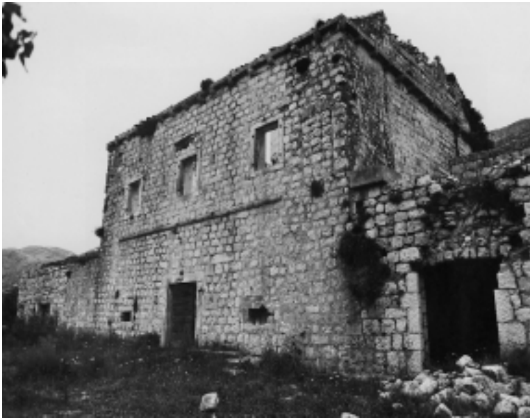
Knežev dvor, južno pročelje s vidljivim bastionskim skošenjem bočnih fasada u prizemnoj zoni, razdjelnim vijencem, puškarnicama i zazidanim ulazom u srušenu ugaonu stražarnicu na prvom katu (foto Miljenko Mojaš) Governor's house, south facade with visibly slanting lateral bastion walls in the ground floor area, cornice, embrasures and walled-up entrance to destroyed corner sentry box on the first floor (photo Miljenko Mojaš)
