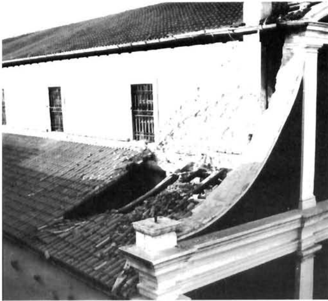
Zadar, Crkva sv. Šime, 5. - 13. st., krov sjeverne lade (foto: P. Vežić) Zadar, St. Simon Church, 5th - 13th c., the roof over the north aisle (photo: P. Vežić)
