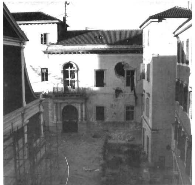
Zadar, Kneževa palača, 13. - 19. st., oštećenja u pročelju (foto: P. Vežić) Zadar, Regent's palace, 13th - 19th c., damage on the facade (photo: P. Vežić)
