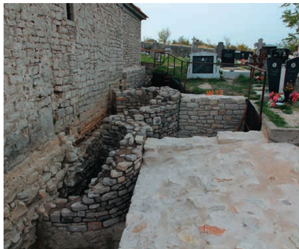
sl. 31. Konzervirani i rekonstruirani W17 (A. Milošević). Fig. 31 Conserved and reconstructed W17 (A. Milošević).
