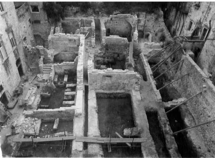
Osnovna škola Grad, vrt s iskapanim novim prilazom (foto: Krešimir Tadić) »Grad« Elementary school, garden with excavation of a new passage of access (Photo Krešimir Tadić)
