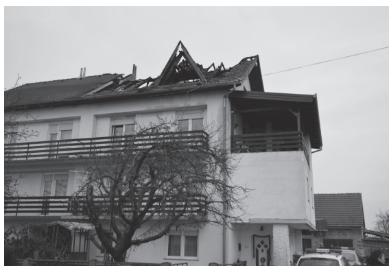
Slika 6. Opožareni objekt prije očevida Figure 6. Building after fire and before investigation
