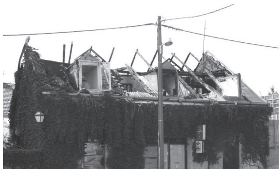
Slika 7. Opožareni objekt Figure 7. Building after fire
