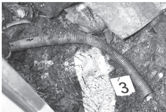
Slika 8. Metalna fleksibilna cijev s tragovima progaranja Figure 8. Metal flexible tube with evidence of burning through the material
