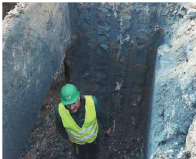
Figure 10. Trial excavation for checking penetration of plastic concrete mix into the surrounding soil
