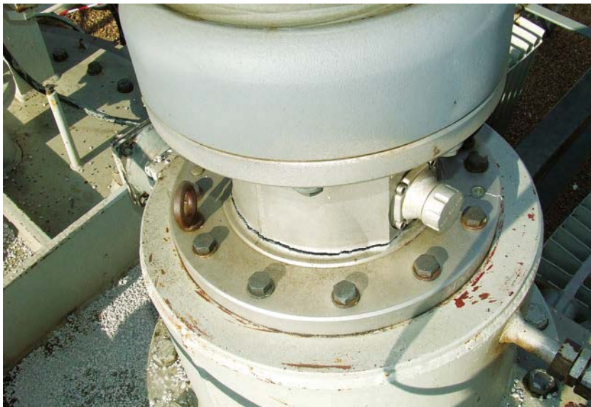
Figure 8. b) Improper gasket sealing in the bushing
