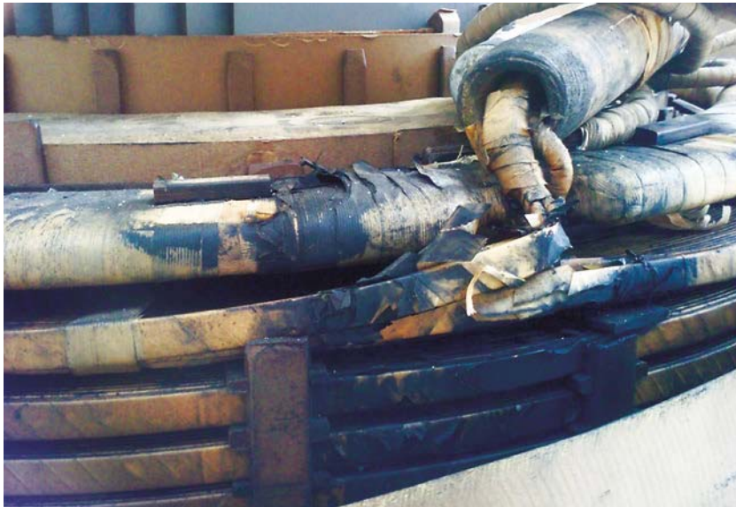
Figure 8. a) Winding damage due to insulation failure
