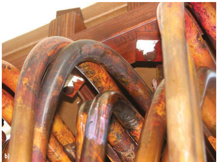
Figure 4. a) and b) Defects in pre-energizing stage appear 3 years after energizing in a furnace transformer of 80 MVA rating
