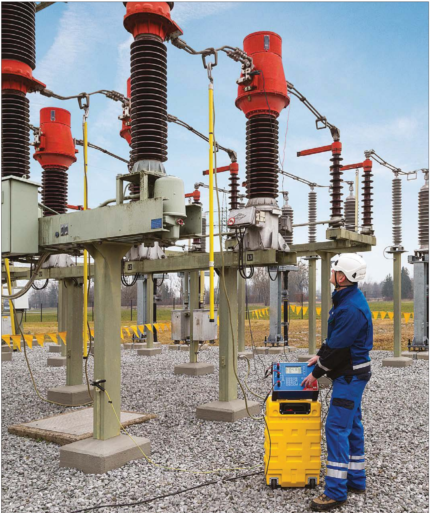
Figure 3. The model-based approach enables automatic assessment of the instrument transformer within seconds
