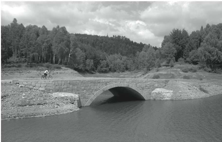
Picture 11. Renovated bridge on the part of the Lujzijana road flooded by the lake. The bridge, Carov most , is visible when the water level is low (Černicki and Forenbaher 2012: 160)
