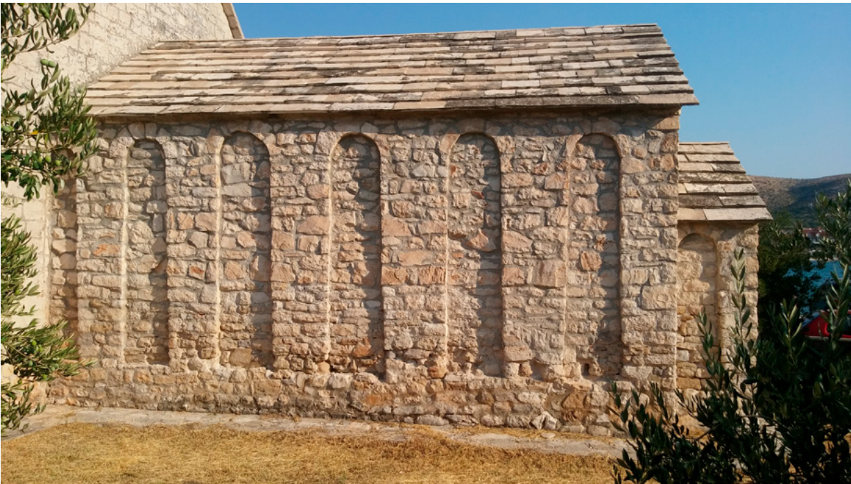
19. Crkva Gospa kraj Mora, sjeverna fasada (fototeka HRZ-a, snimio P. Gamulin, 2019.) Church of Our Lady by the Sea, north façade (Croatian Conservation Institute Photo Archive; P. Gamulin, 2019)
