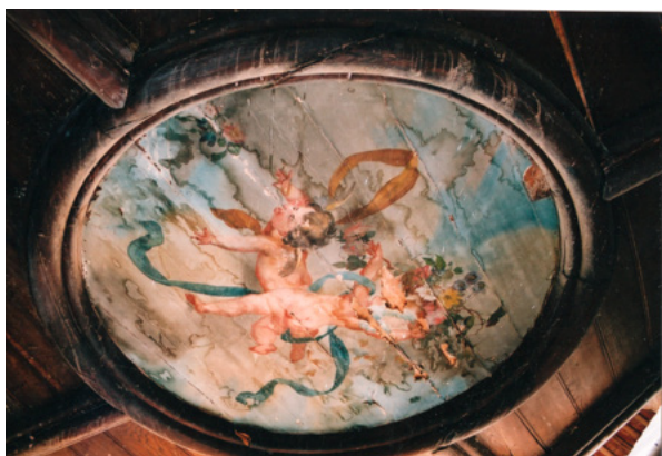
5. Jedan od medaljona nakon urušavanja krovišta i stropa dvorca (fototeka MK RH, KO Zagreb, snimio N. Bradić, 2003.) One of the medallions after the collapse of the manor house roof and ceiling (Ministry of Culture of the Republic of Croatia, Conservation Department in Zagreb Photo Archive; N. Bradić, 2003)
