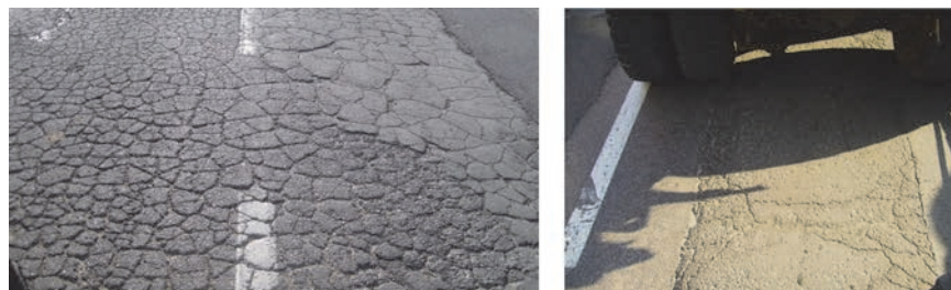
Figure 7. Net-alligator cracks of high intensity (left side) and patches of medium intensity (right side)
