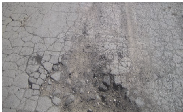
Figure 8. High intensity pothole adjacent to net-alligator cracking
