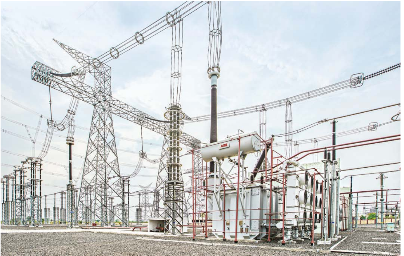
Figure 4. 1200 kV AC Power transformer at the substation in India
