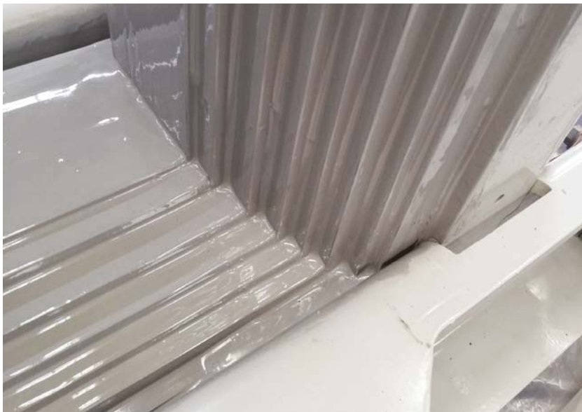
Figure 7. All core parts should be completely covered with the paint layer, especially the areas that are hard to reach such as corners or tight spots
