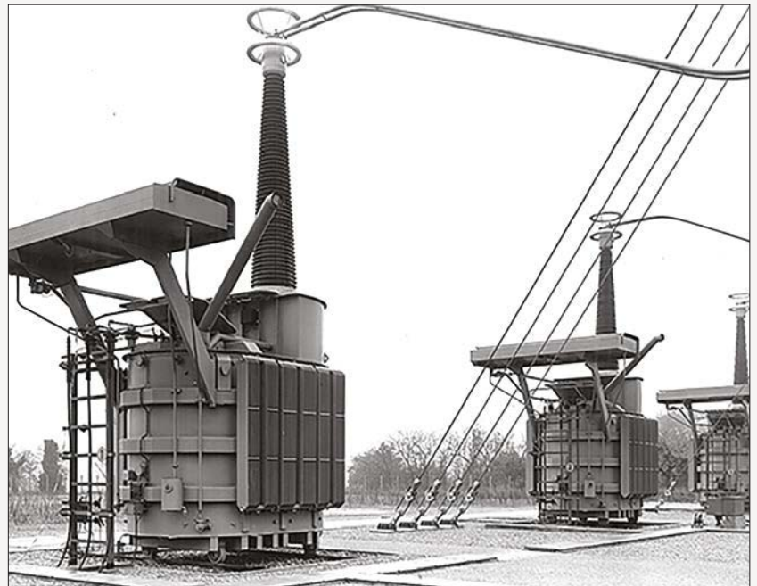
Figure 5. GE's first 1,050 kV transformer for extra-high voltage test lines in the 1960s
