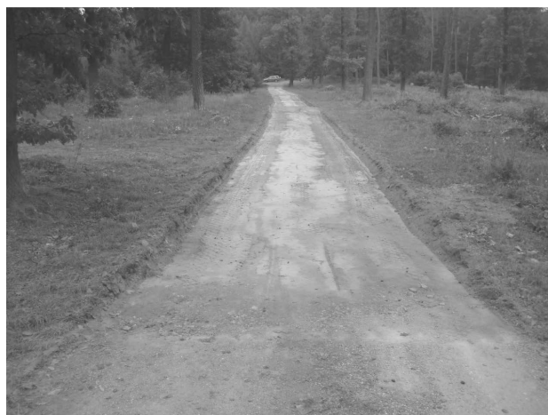
Fig. 1 Removed original subgrade (seen at the front of the picture) and preparation of new subgrade for new surfacing
