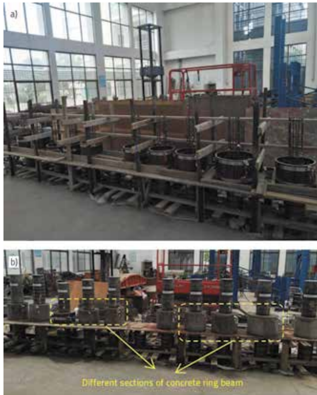
Figure 3. Specimen manufacturing process: a) Placement of reinforcement skeleton; b) PRB and PCR
