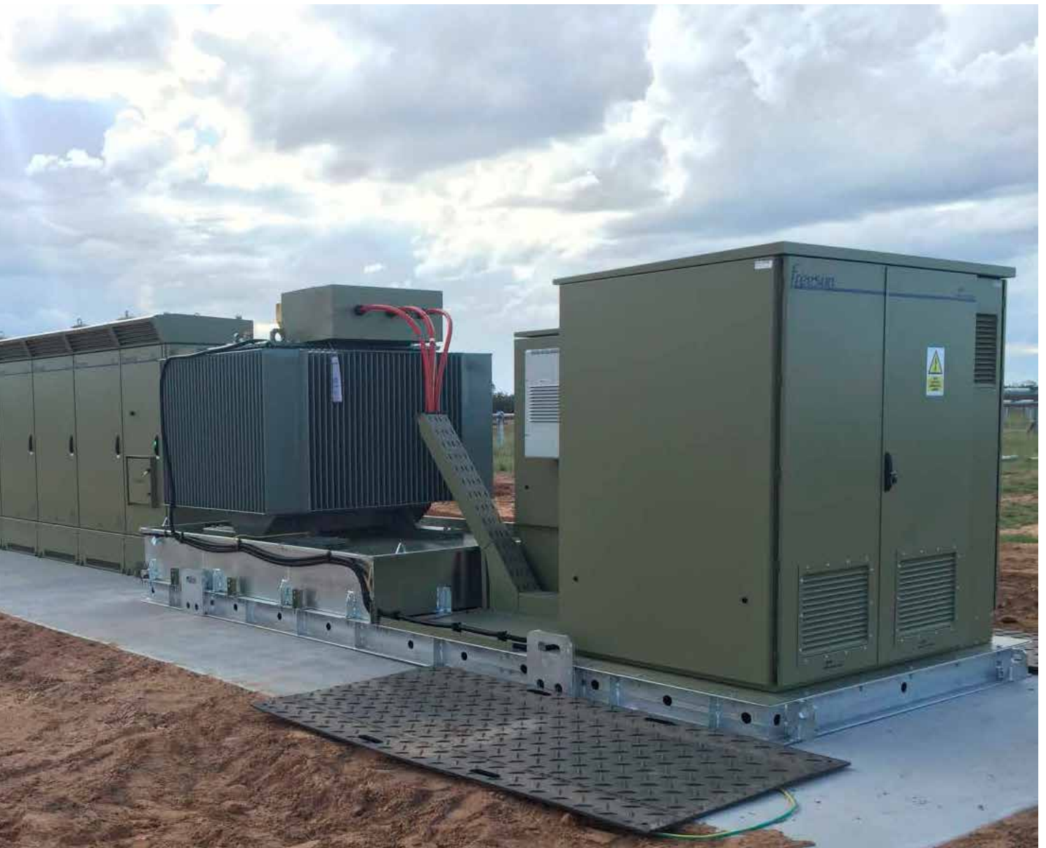
Figure 1. 2.5 MVA transformer/inverter package with MV switchgear [1]
