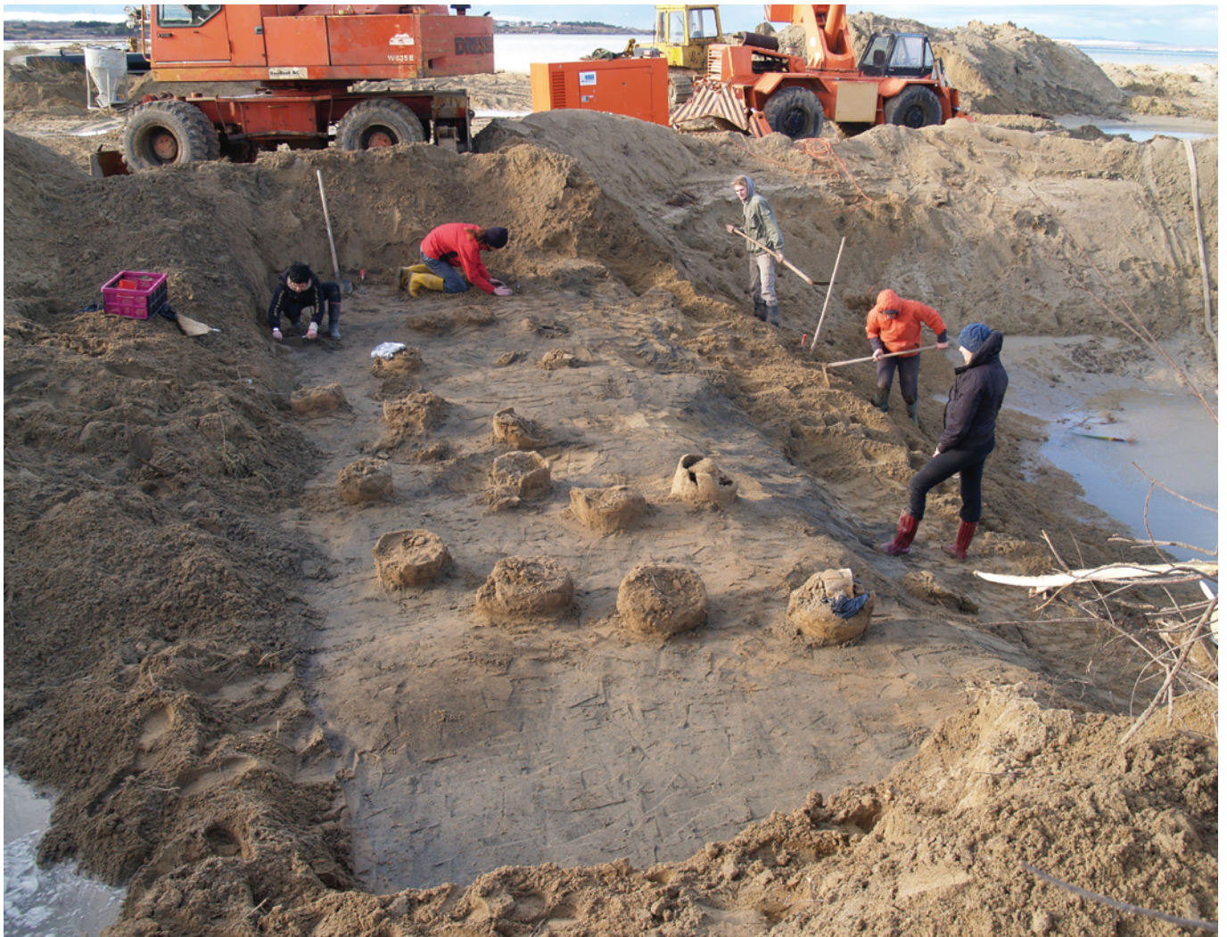
Slika 6. Pogled na sjeverni dio sonde tijekom rada Figure 6. View of northern part of trench during excavations
