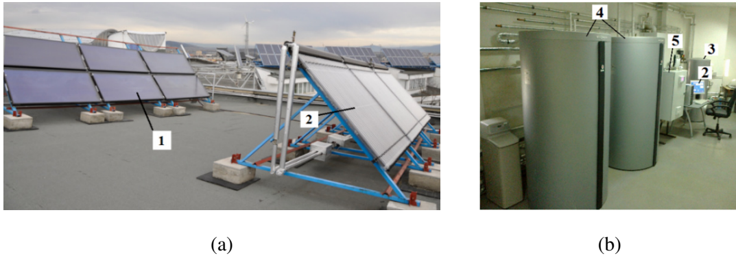
Figure 2. Solar thermal system installed in the in the Colina Campus of RESREC Research Centre: solar thermal collectors installed on the rooftop (a) and storage tanks, controllers and monitoring system installed in the laboratory (b)
