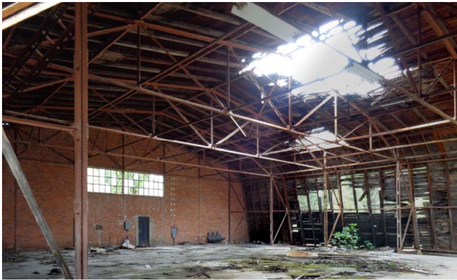
Figure 18. Hangar no. 3 with shell hit. The brick-built back wall does not belong to the original hangar construction (M. Martinović)
