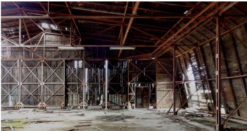
Figure 16. Type In hangar (no. 3) in Mostar: the iron frames and rails for the sliding door elements are intact (M. Martinović)
