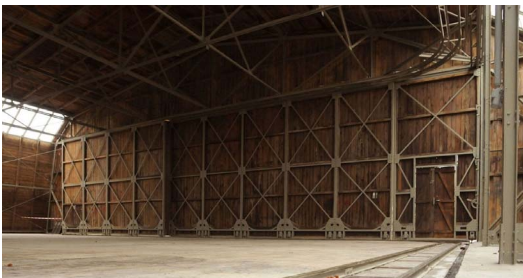
Figure 17. Vision for the re-establishment of the Mostar hangars. The Krakow hangar still lacks a wooden floor, so the door rails raise over the floor horizon
