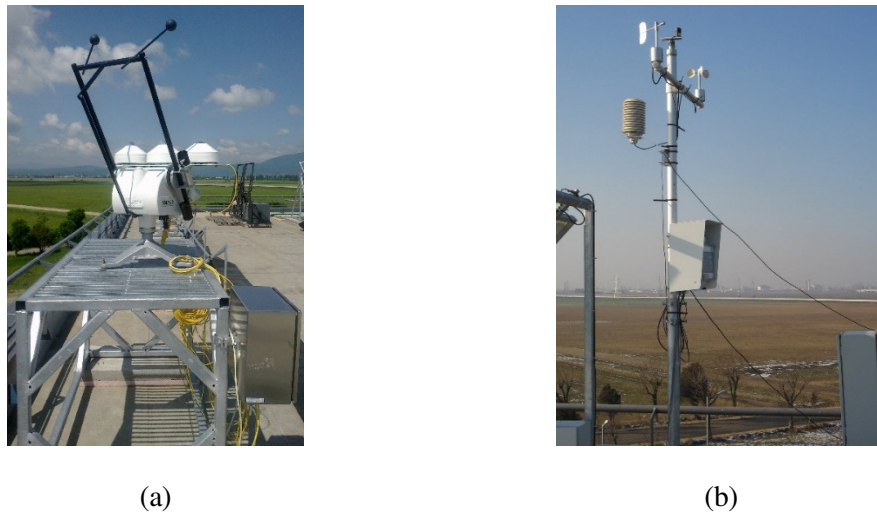
Figure 2. Meteorological parameters monitoring system: Solys2 Sun tracker (a) and DeltaT weather station (b) installed on the laboratory rooftop
