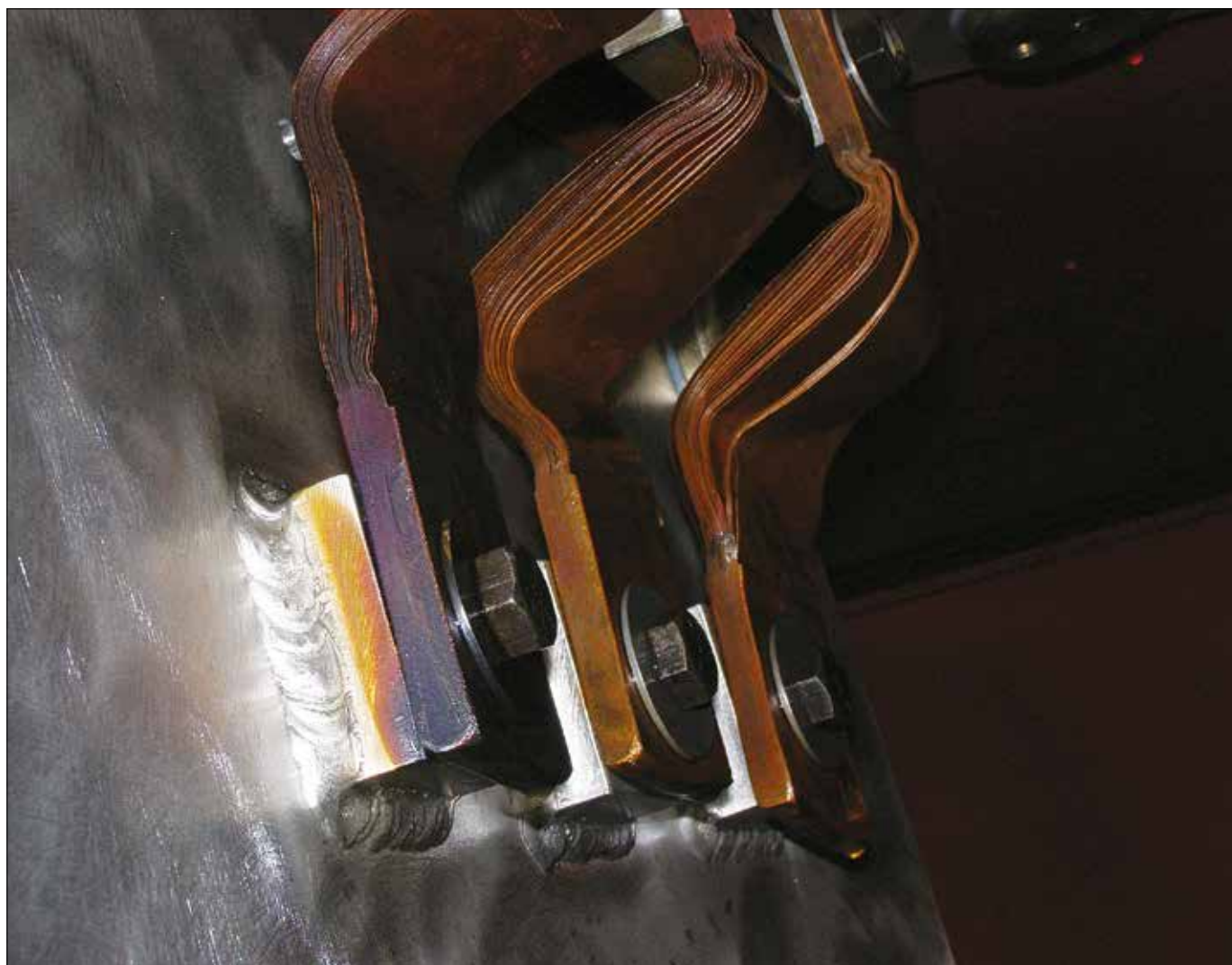
Figure 5. DGA signal created by sulfur corrosion phenomena, ethylene reaches 750 PPM
