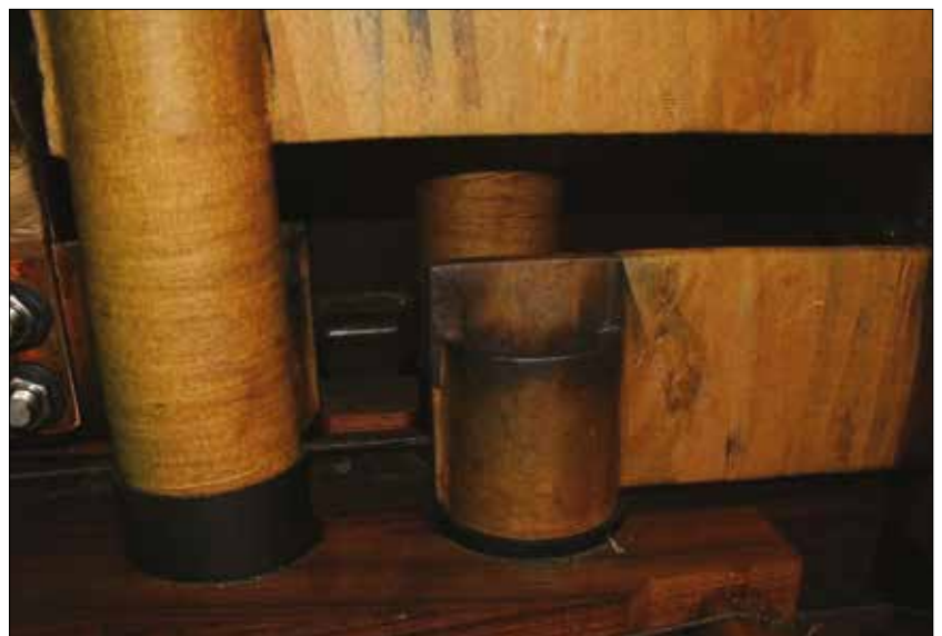
Figure 4. Sulfur corrosion phenomena for a step-up transformer energised with original oil since 1960
