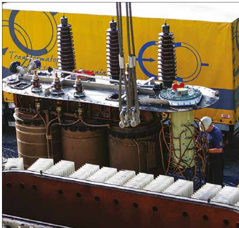
Figure 6. View of the active part of the transformer during renovation on site
