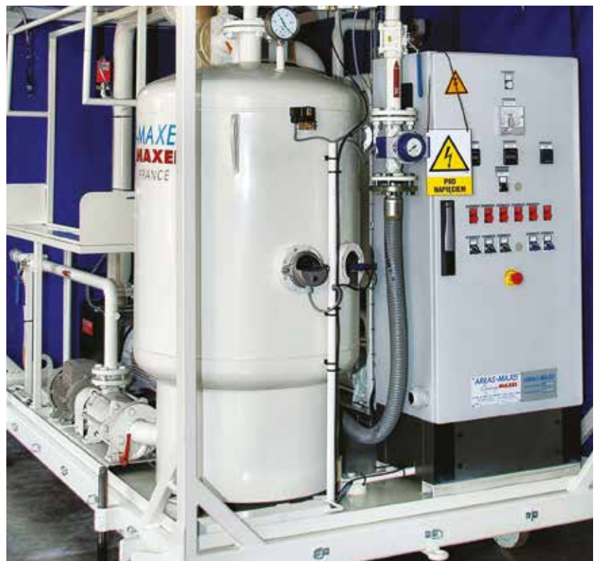
Figure 2. View of the device for regeneration and treatment of insulating oil
