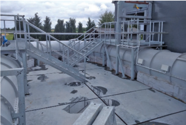
Figure 12 Water tunnel Slika 12. Vodeni tunel
