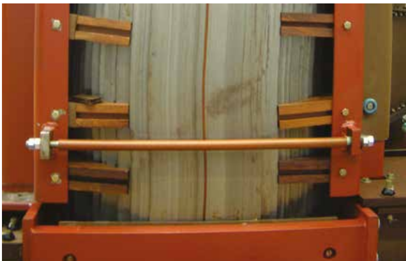
Figure 2. Transformer critical failure without any DGA signal alarm
