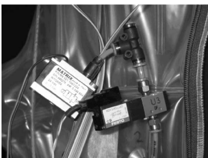
Fig. 18 The electromagnetic valves for filling and releasing compressed air into the thermoinsulating chambers with a part of the air duct system and the T-plug connection
