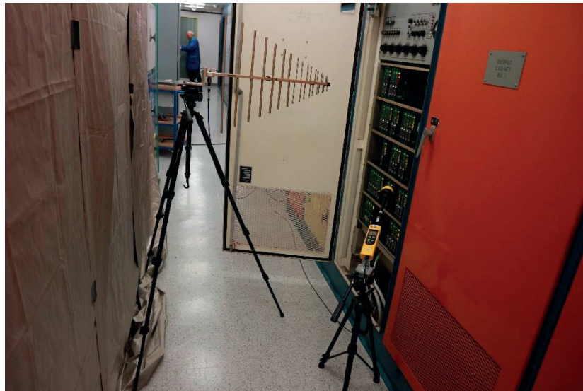
Figure 1 Immunity Test of Solid State Protection System (SSPS) Cabinet in MCR
