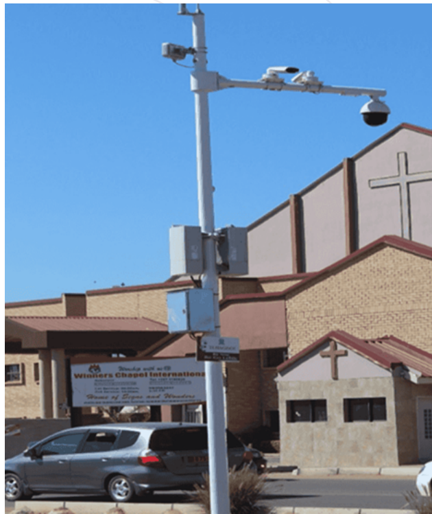
Image 3. CCTV that had a warning label attached in Block-6. Photo: S. Molepo.
