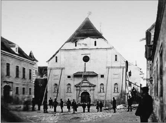
SL. 4. UČVRŠĆIVANJE OŠTEĆENOG PROČELJA CRKVE SVETE KATARINE NAKON POTRESA (FOT. HERMANN FICKERT, 1880.) FIG. 4 BRACING THE EARTHQUAKE-DAMAGED FACADE OF THE CHURCH OF ST. CATHERINE (PHOTO BY HERMANN FICKERT, 1880)
