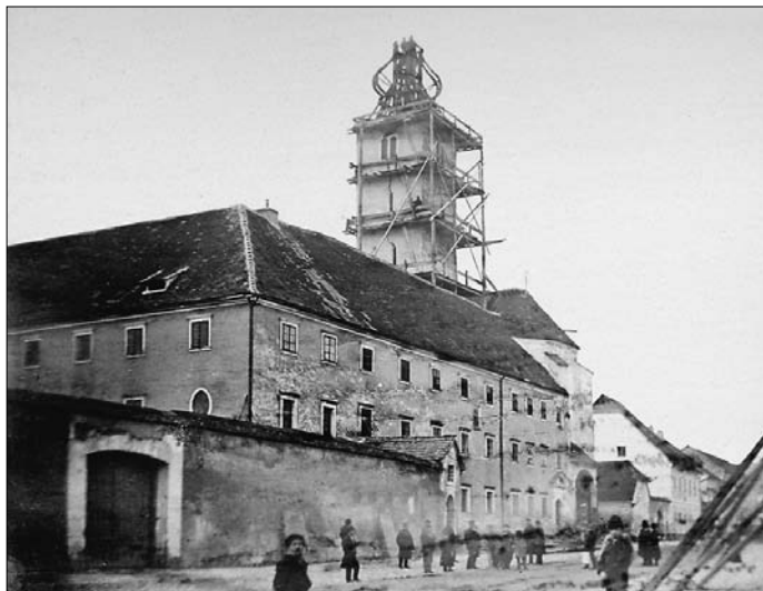
SL. 15. UKLANJANJE TORNJA FRANJEVAČKE CRKVE U STUDENOME 1880. (FOT. HERMANN FICKERT, 1880.) FIG. 15 REMOVING THE TOWER OF THE FRANCISCAN CHURCH IN NOVEMBER, 1880 (PHOTO BY HERMANN FICKERT, 1880)
