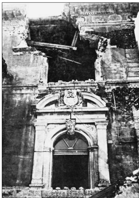
SL. 4. OŠTECENA ZGRADA STARE VIJEĆNICE U STAROM GRADU KOTORU FIG. 4 DAMAGED OLD TOWN HALL IN THE OLD TOWN KOTOR
