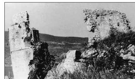
SL 8. OŠTEĆENI SAMOSTAN PODLASTVA U GRBALJU, BUDVA FIG. 8 DAMAGED THE MONASTERY PODLASTVA IN GRBALJ, BUDVA
