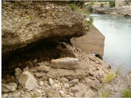
Figure 14. A scoured layer of conglomerate susceptible to collapsing
