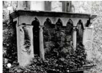
19 Projekt 21: stanje balkona prije radova Project 21: condition of balcony before restoration
