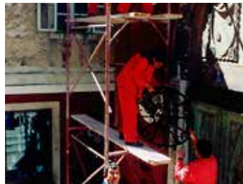
8 Projekt 9: montaža rešetke na pročelje palače Divnić Project 9: installing of metal grating to the façade of Divnić palace
