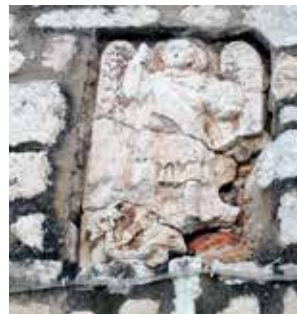
23 Projekt 31: stanje grba prije radova Project 31: condition of coat of arms before restoration
